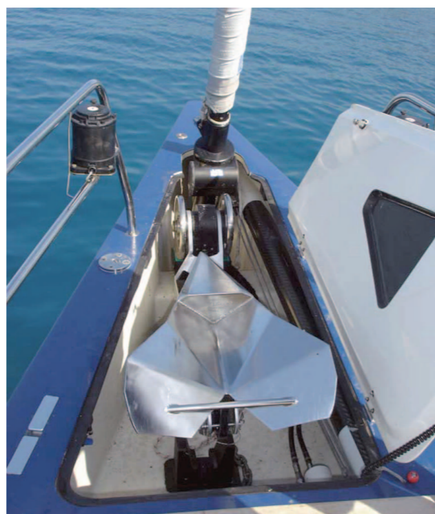
Anchor stowing motor
